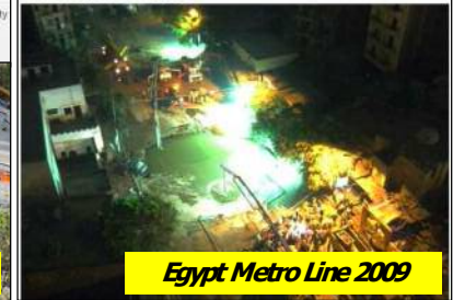
Metro Construction Causes Sinkhole in Downtown Cairo
